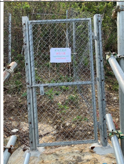
Photo 2 – Current situation of fencing and warning sign
